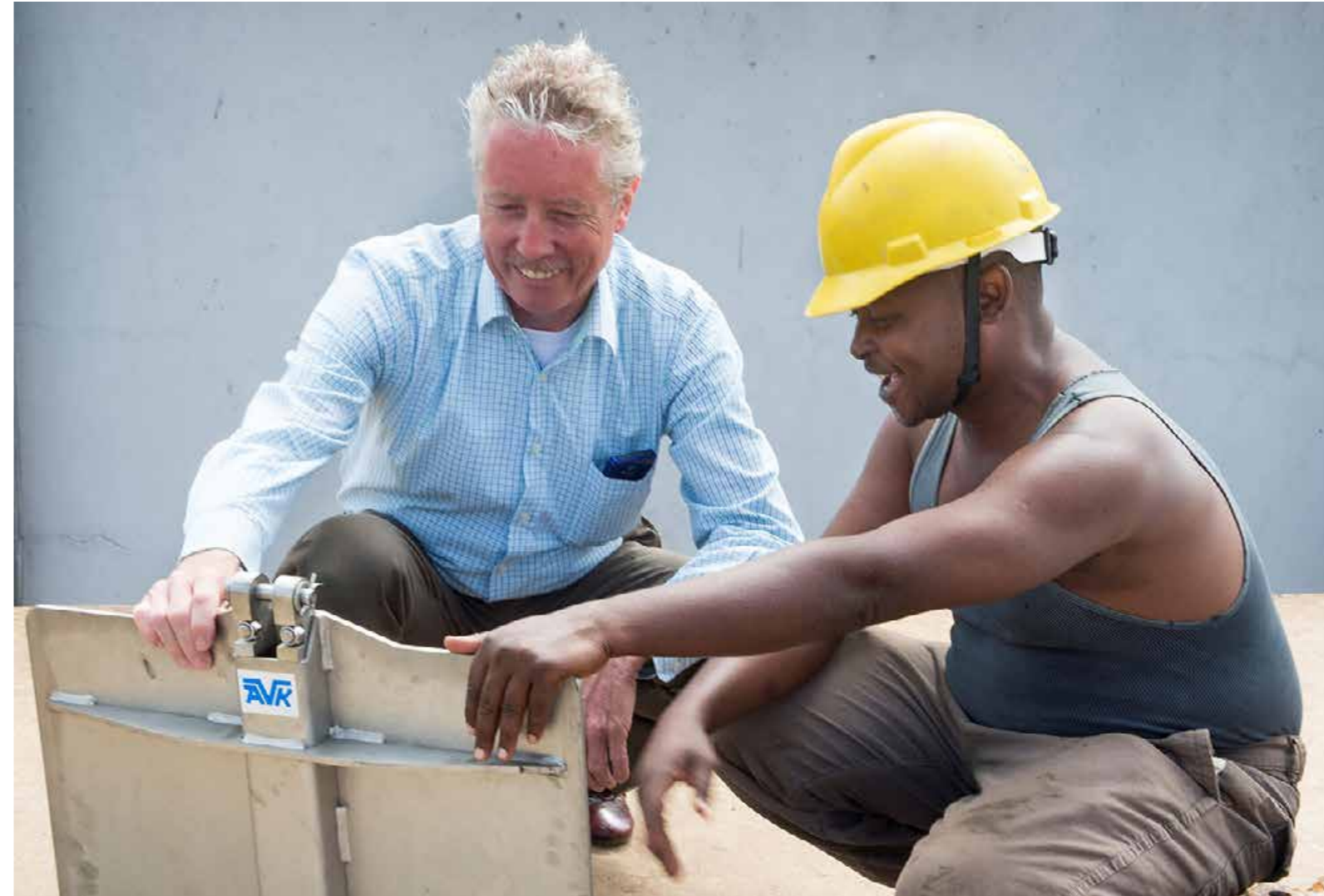
Malawi – Installing new gate valves at Lilongwe Water Board by Project Manager Rob Beckers. Credits: Rob Elfring.
