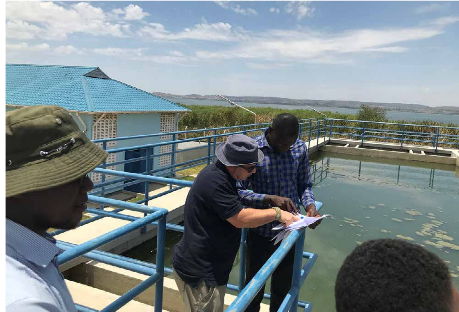
Mwanza – Water treatment plant
