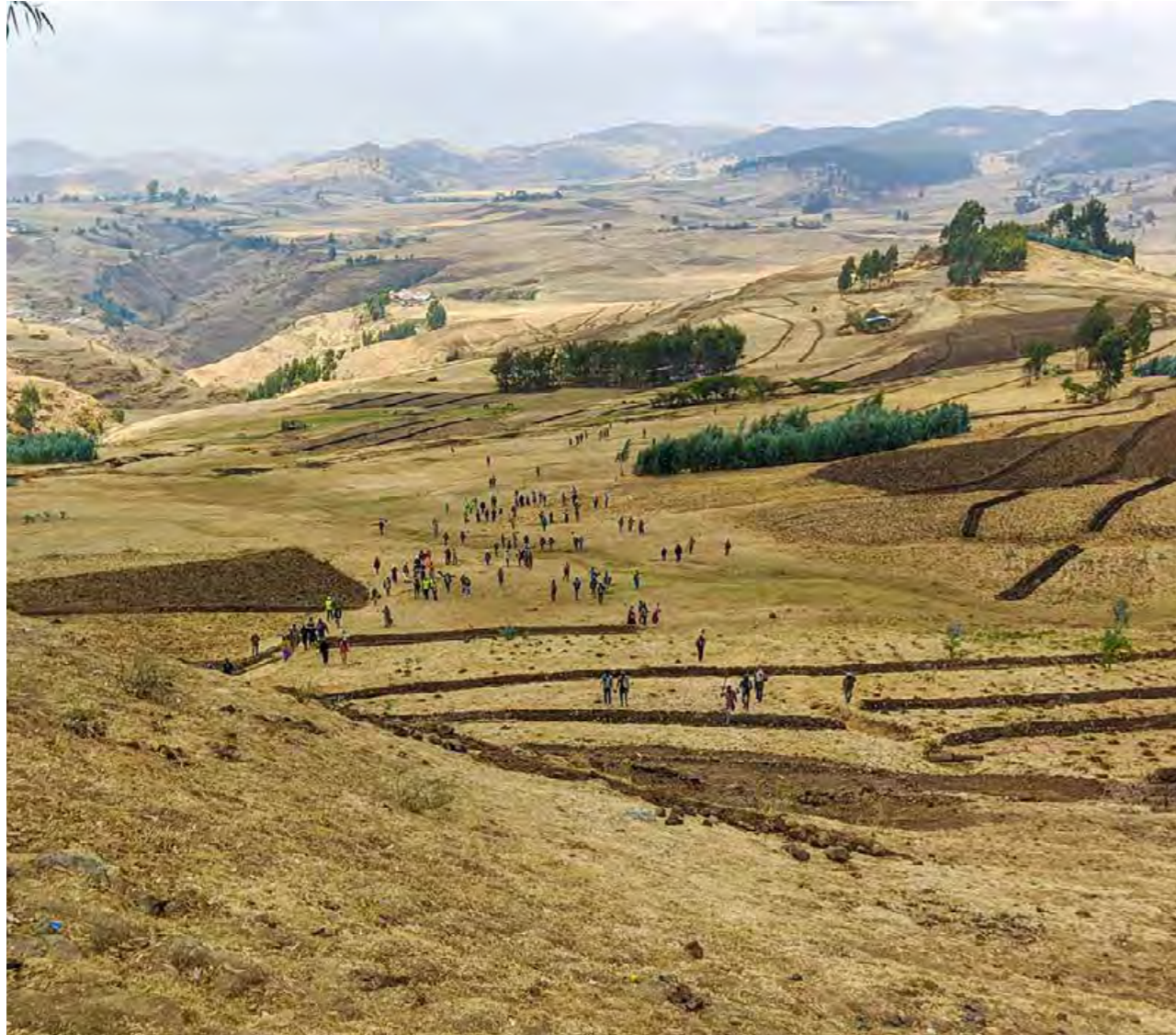
Ethiopia – The Integrated Water Resources Management for Water Sanitation and Hygiene (IWRM4WASH) project with partners Addis Ababa water and Sewerage Authority (AAWSA) and the Oromia Water and Energy Resource Development Bureau (OWERDB).
