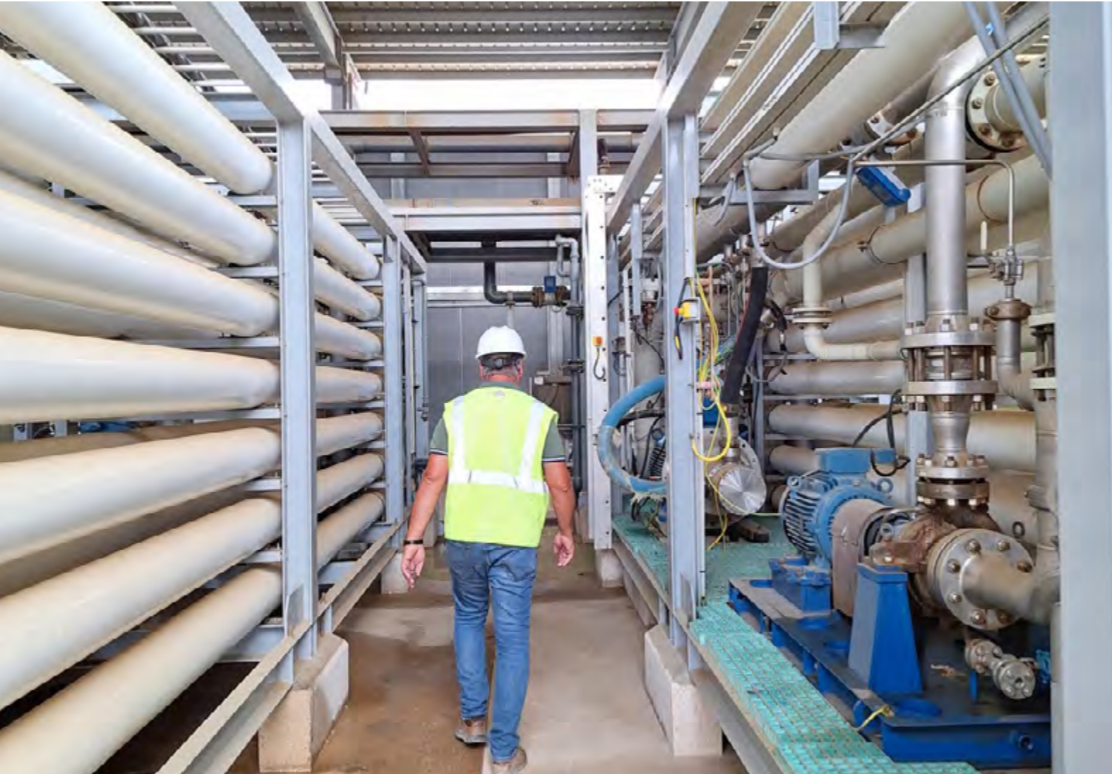
Bonaire – Water Operator Partnership with WEB Bonaire.
