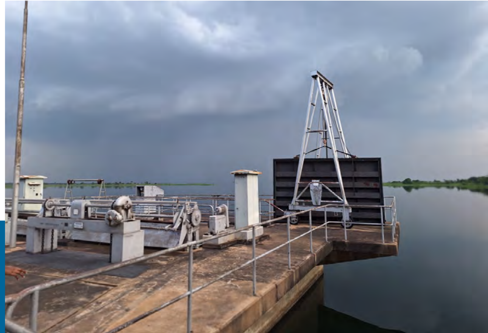
Ghana – Kpong Water treatment plant.
