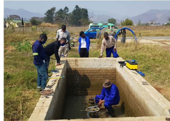
Zimbabwe – Local knowledge exchange from a plumber in Harare explaining to the technical team in Mutare how to set and maintain a pressure reduction valve. This will reduce the high occurring pressures in the mountainous area of Mutare.
