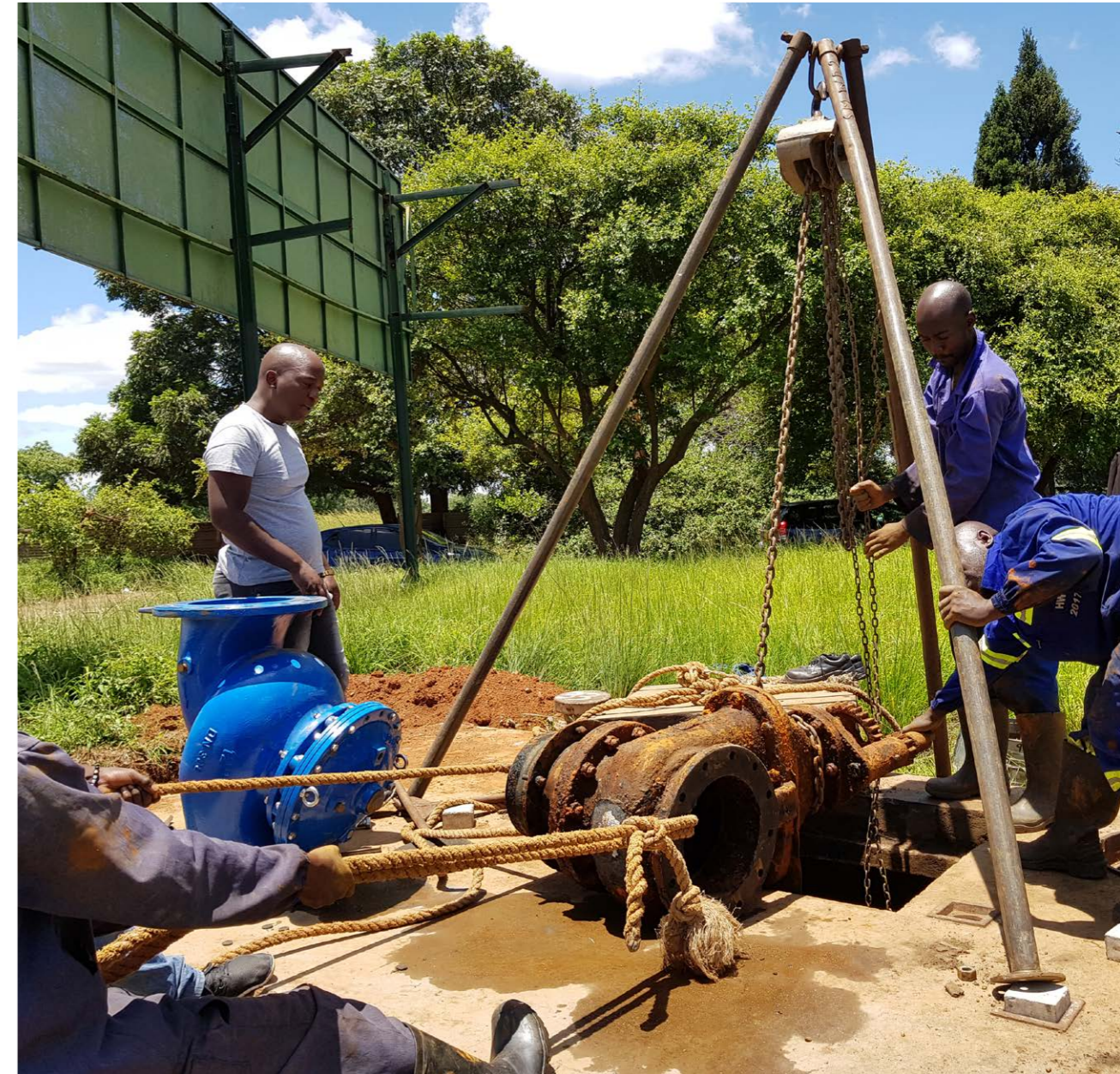
Zimbabwe — Local Young Expert Victor Shana supervising the replacement of a pressure reduction valve, one of the most effective ways to reduce leakage and prevent bursts in Harare.
