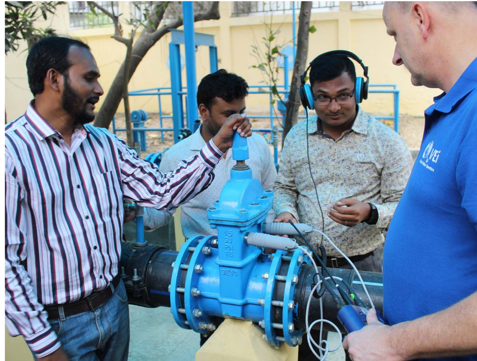
Bangladesh – In the training center built by VEI, District Meter Area managers receive training with the correlator to detect leaks in the pipe network.
