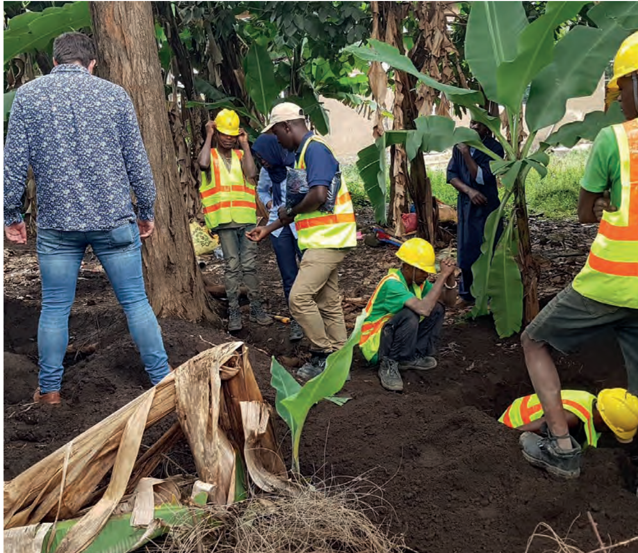
Tanzania – VEI (Jan-Kees de Visser) supporting to disconnect the old network in Arusha City Centre from the newly laid network by the African Development Bank, resulting in reduced Non-Revenue Water.
