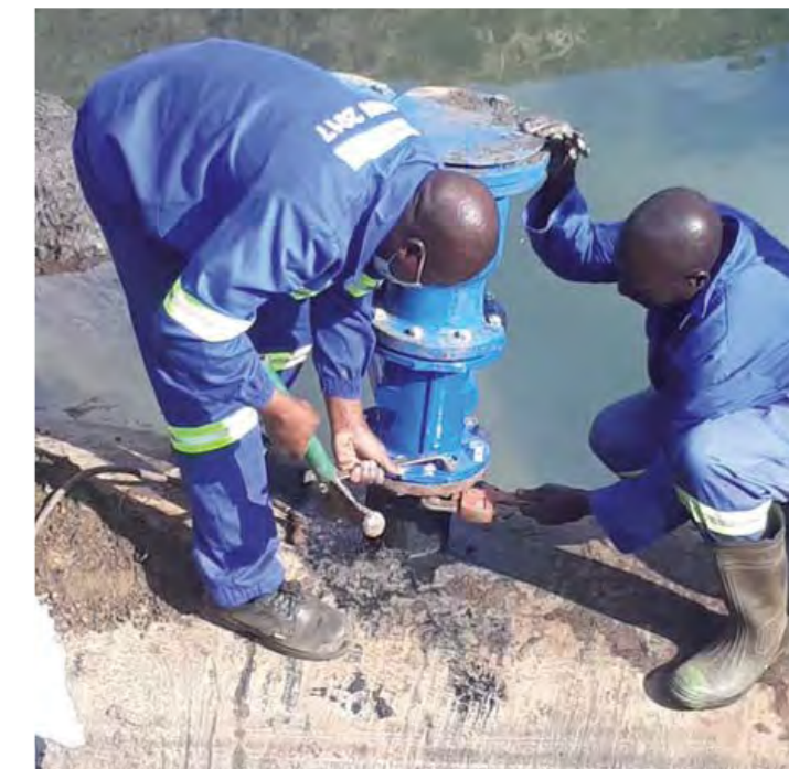
Zimbabwe – Leak repairs as part of the Harare emergency program to fight the cholera outbreak.
